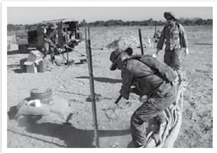
Leading Aircraftmen David Clewes (front) and Matt Larkin constructing latrines at Comoro, September 1999 – Facilities were initially basic but progressed
