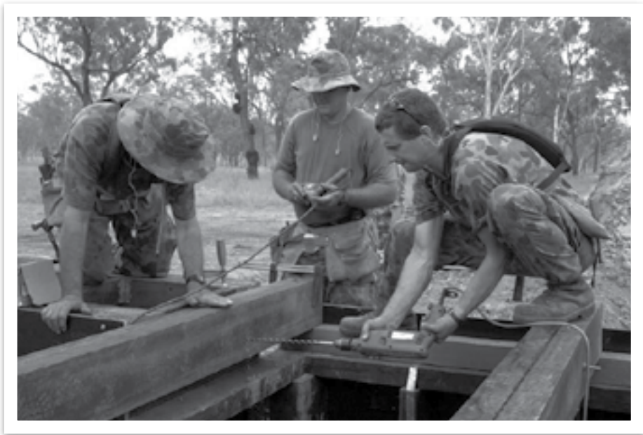
Leading Aircraftmen Bevan Gillam (right) and Mark Fellows (centre) build a hardened command post, High Range, Townsville, 2004 – Command for the home bases changed four times in five years
