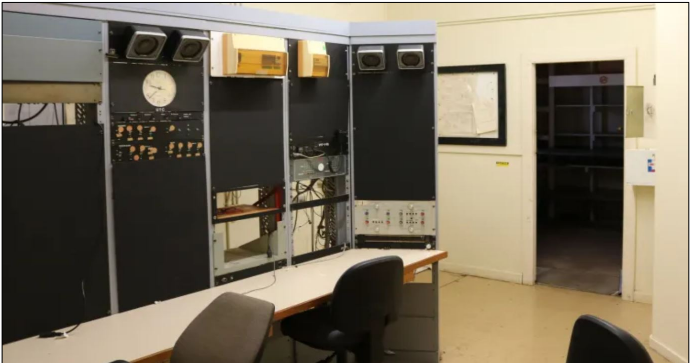
The interior of the receiving station. Unfortunately all the original equipment has long since gone but there are a number of signs in the building showing what was once what. Click each sign to be able to read it..
